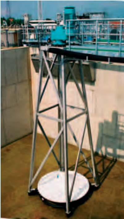
1 out of 9 HYPERCLASSIC®-Mixer/Aerators in an industrial wwtp in Belgium (Pulp & Paper Industry)
