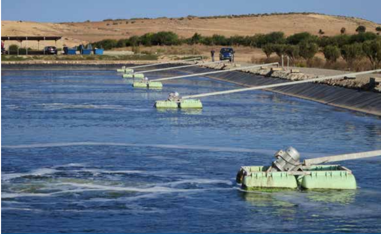
OxyStar® aerators on floats in a wastewater lagoon (Morocco)
