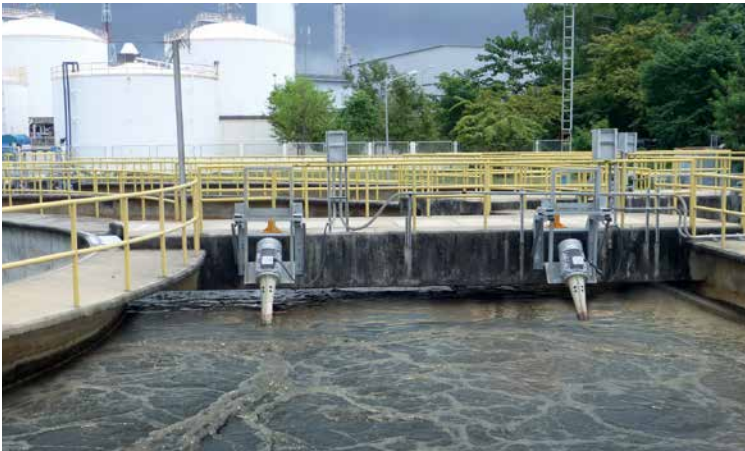
Activated sludge tank of an industrial sewage treatment plant (Thailand)
